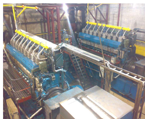
Figure 5 - View of the two engines 9L32
