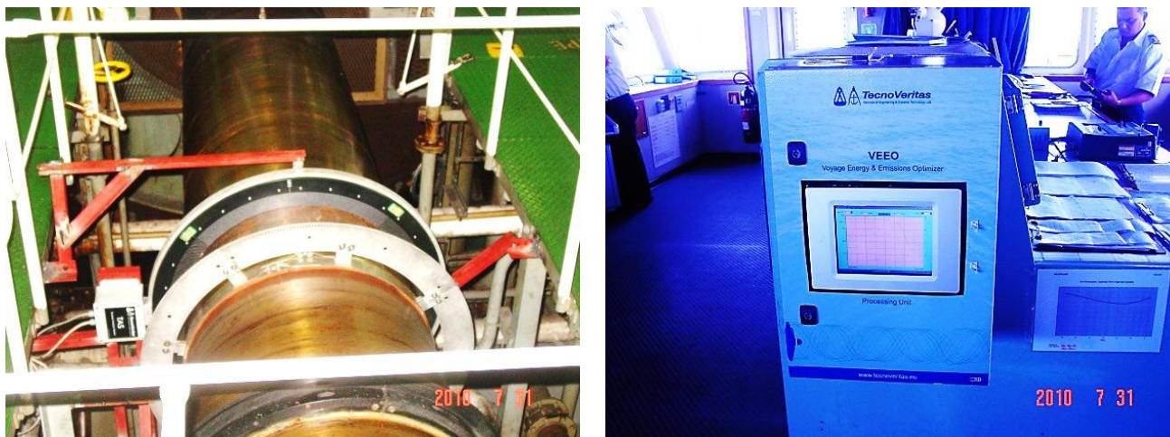
Figure 5 - Bridge VEEO cabinet and shaft torque.
