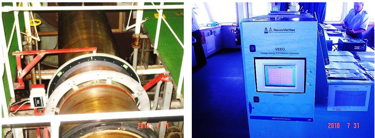
Figure 5 - Bridge VEEO cabinet and shaft torque.
