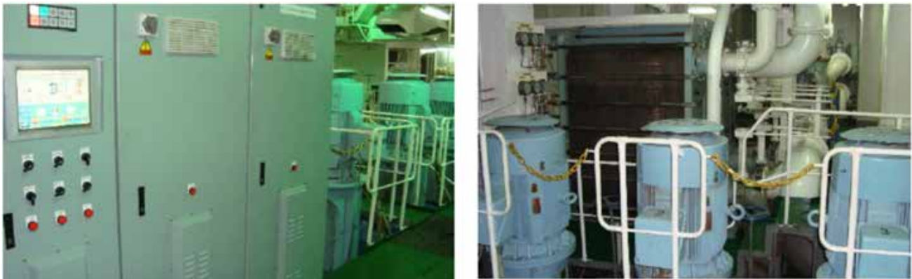
Figure 9 - Aspect of the SW circulation cooling pumps and respective Variable Speed Drives (left).
