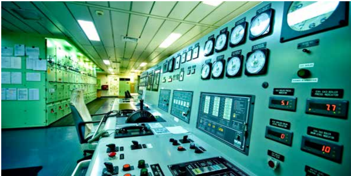
Img 1. Expensive control and monitoring systems, need to be complete.
