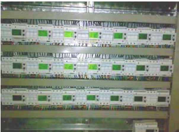
Img. 1 | System analysis of energy consumption mounted Central Trigeneration Climaespaço in the Park of Nations in Lisbon (installed in 2009)
