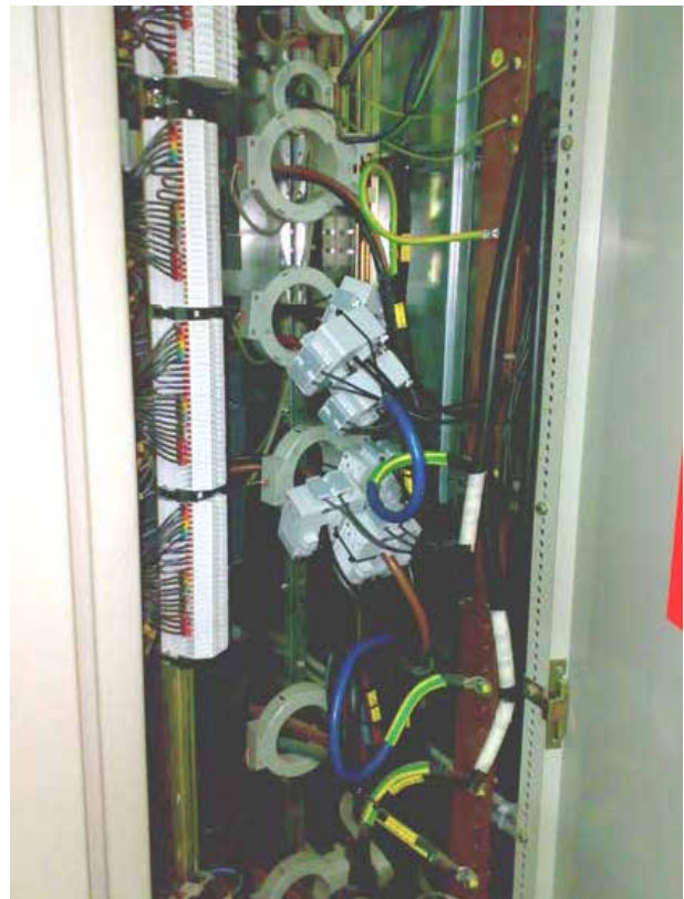
Img. 2 | Ti's frame mounted on Climaespaço Center Trigeneration (installed in 2009).
